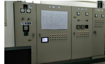
▲ PLC Control Panel of the Wastewater Treatment Plant
