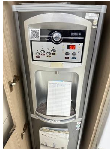
▲ Monthly Drinking Water Dispenser Maintenance Records
