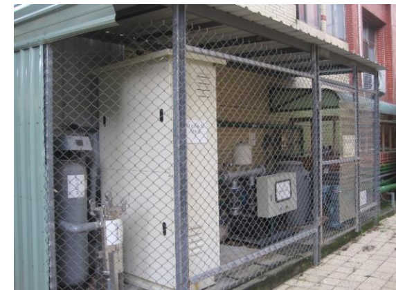
▲ Rainwater Harvesting and Reuse System
